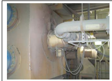
Burner end of dryer with natural gas and combustion air piping
