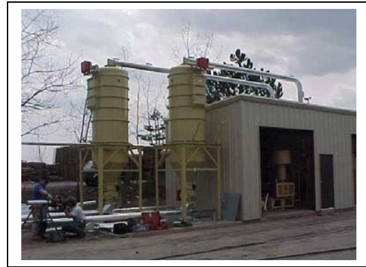
Vacuum Receivers and pump house along rail siding
