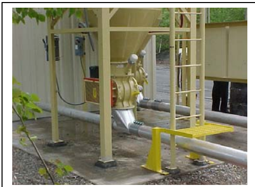
Airlock under vacuum receiver connecting to pressure conveying system
