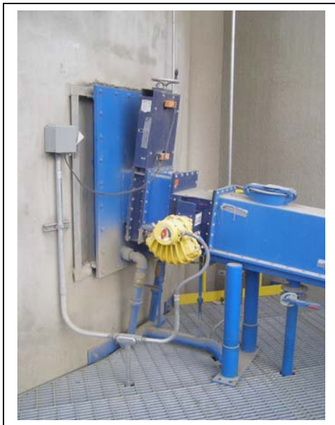
External view of silo penetration feeding closed air slide
