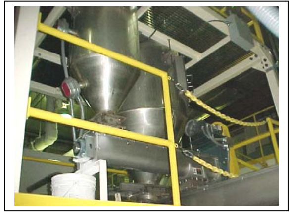
Two vacuum receivers mounted in a steel structure
