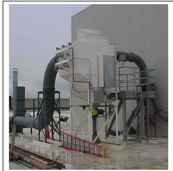
Roof top dust collector with explosion vents
